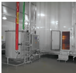
Full recirculating cleaning system
