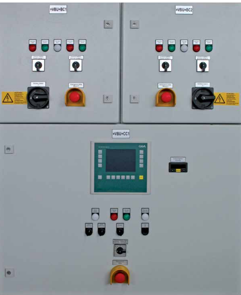
Control Panel with PLC
