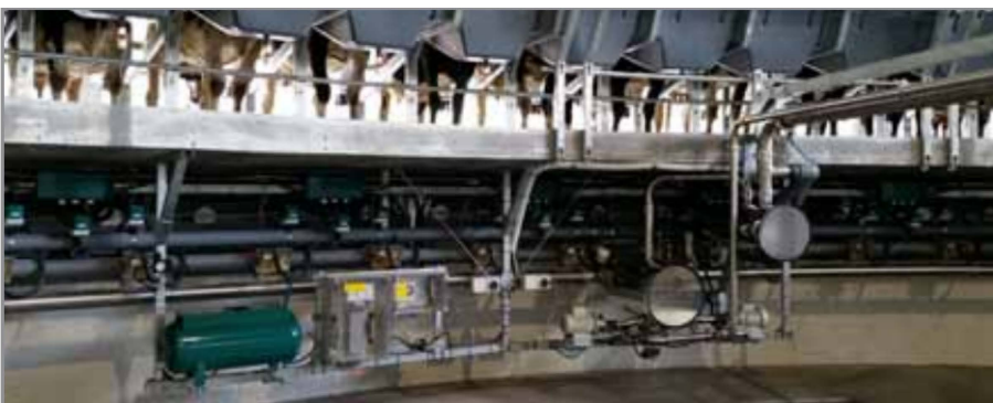
Left: Integrated solution using Milfos iFLOW platform with Westfa/iaSurge milking equipment.
